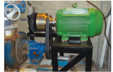
Flux Drive® Sheave ASD belt-driven installation with raised motor foundation.
