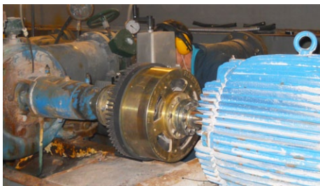
A Flux Drive® Adjustable Speed Drive installed at the Vancouver Aquarium Wild Coast Exhibit
