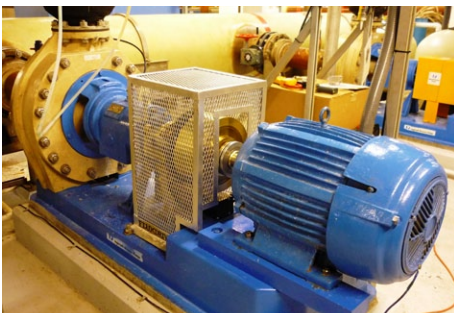
Flux Drive ASD Model 10 – 150 (50 hp) filter pump application at Moody Gardens
